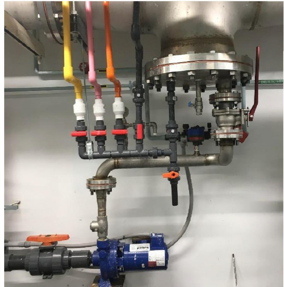
Figure 4.5 Flash Mixer (Prior to Alum Dosage System Upgrade) 2023-10-28
